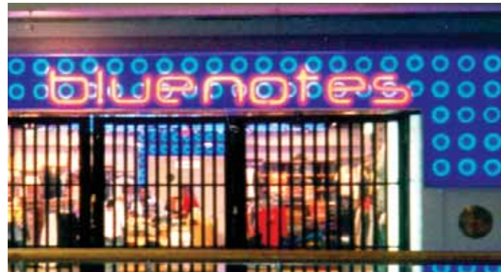
Unacceptable - exposed neon tubes
