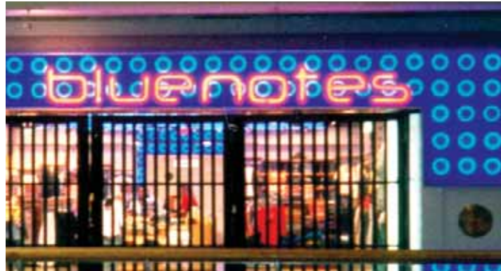
Unacceptable - exposed neon tubes
